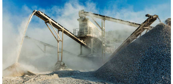
Rock crushers can spray water to control PM emissions.
