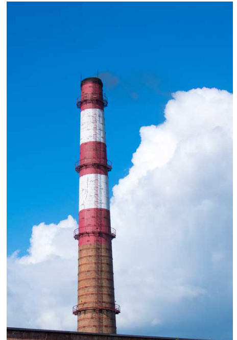
Lime injection into exhaust gas helps absorb SO 2 before release from tall stacks.
