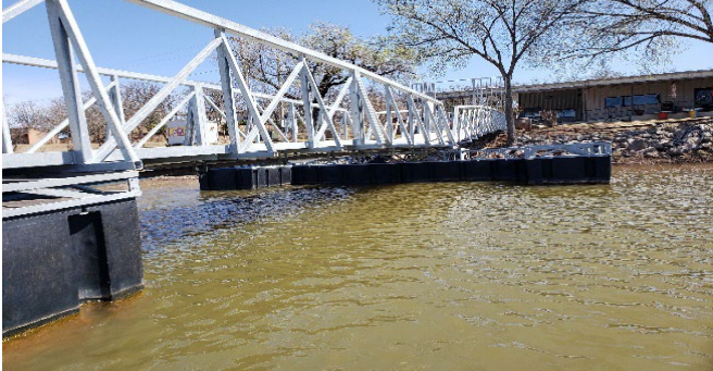
Photo Series #4. Calypso Cove Marina on Lake Thunderbird. April 1, 2022. Brand new marina dock and piping to connect the pump-out station and lift station.
