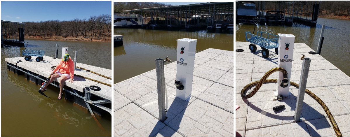
Photo Series #2. Calypso Cove Marina on Lake Thunderbird. April 1, 2022. Demonstration pump is running properly. Newly installed pump-out station. Brand new marina dock.
