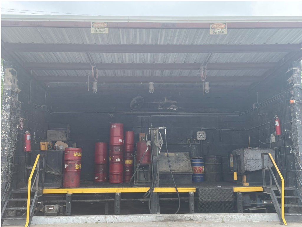
Figure 5: Return and Fill Station
